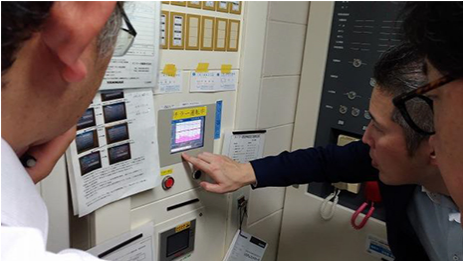
Energy consumption diagnosis at SS30
