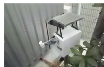
Example of water conservation equipment: Water sprinkler equipment at Luz Jiyugaoka
